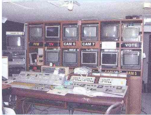
Parliamentary Meeting System and Closed Circuit Television Control Room
